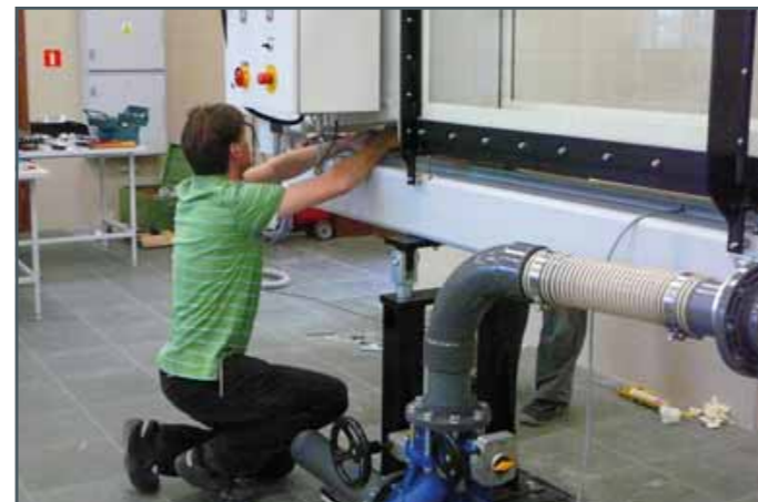
Last but not least is work on the wiring (left). Then the water tank is aligned and connected to the pipeline system (right).
