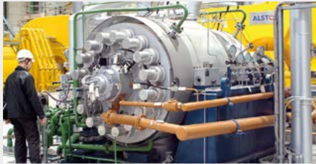
A centrifugal pump at a power plant
