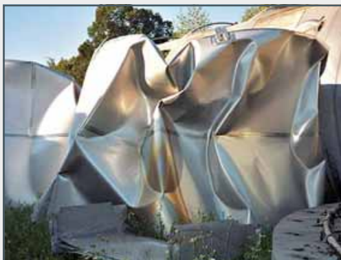
Collapsed tank as a result of water hammer
