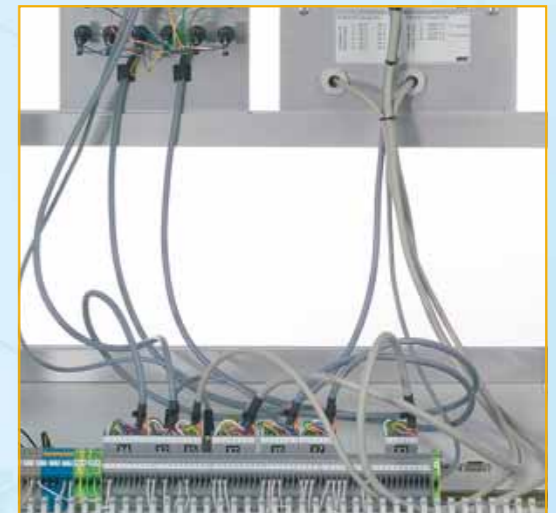
Industry-standard, flexible cabling
