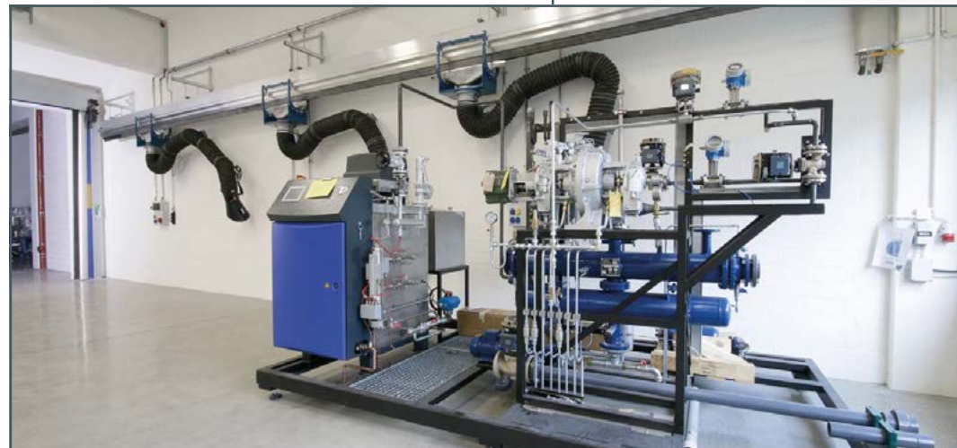
Exhaust gas extraction for combustion engines and steam generators
